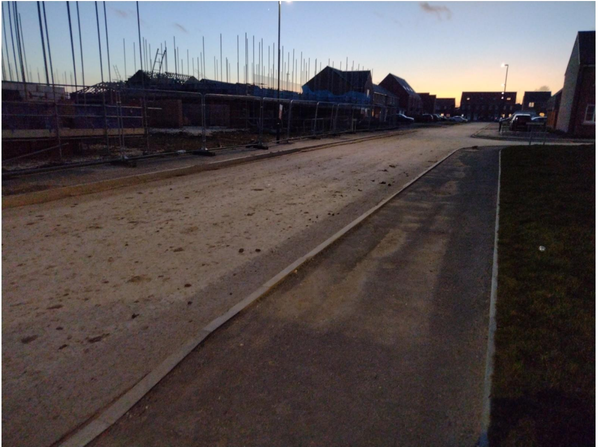
Albertross Drive to Eagle Drive taken from our Driveway – again no road sweeper used – taken 31 st January 2022. No hoardings to cover the works.
