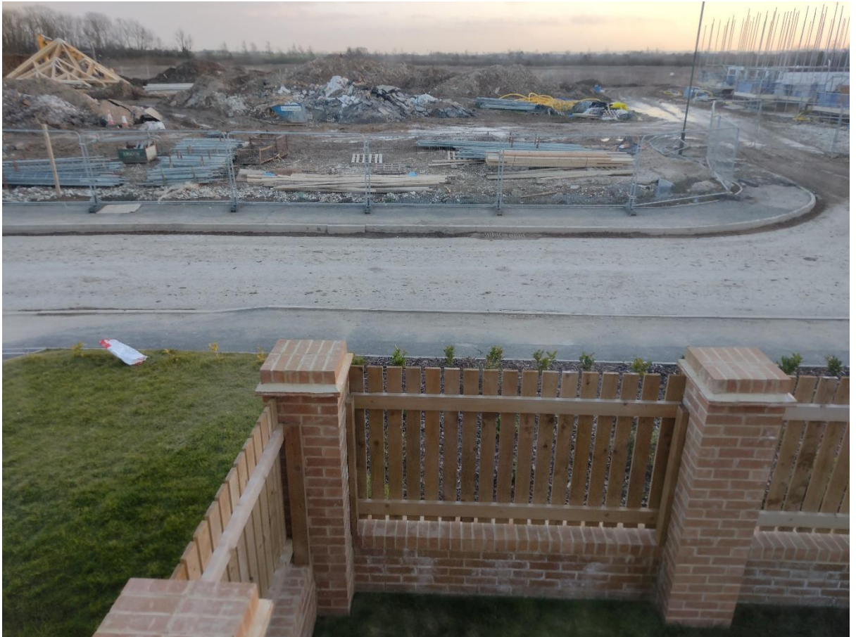
Used to at least be Persimmon hoardings on the fence to cover the works but no longer it seems – more litter in our garden from the estate
