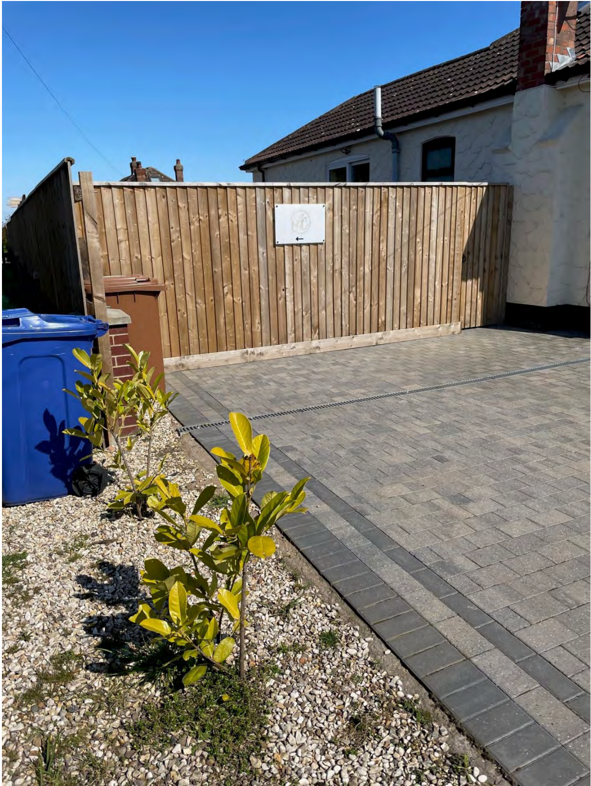
Side fence that attaches to boundary fence with Side Lane. This was at back of bungalow as plans show but moved to front of bungalow therefore parking and turning area greatly reduced . Plans are incorrect
