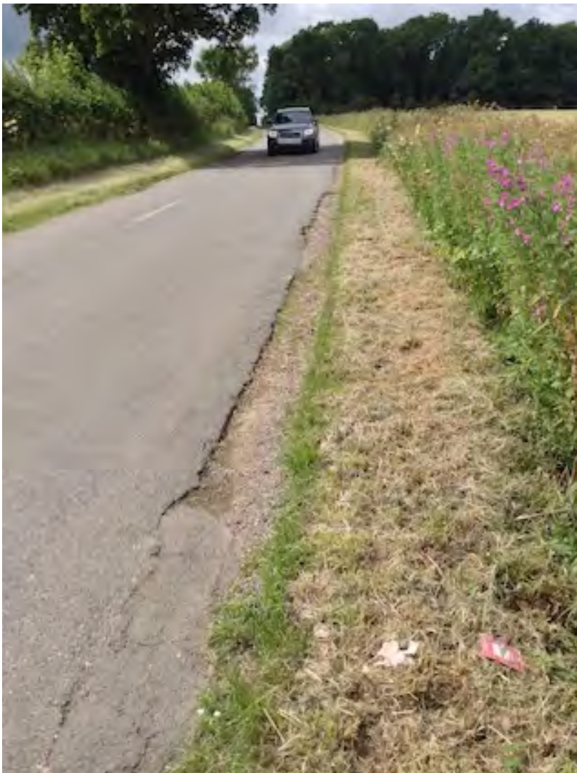
Traffic forced into centre of road due to crumbling road edges.
