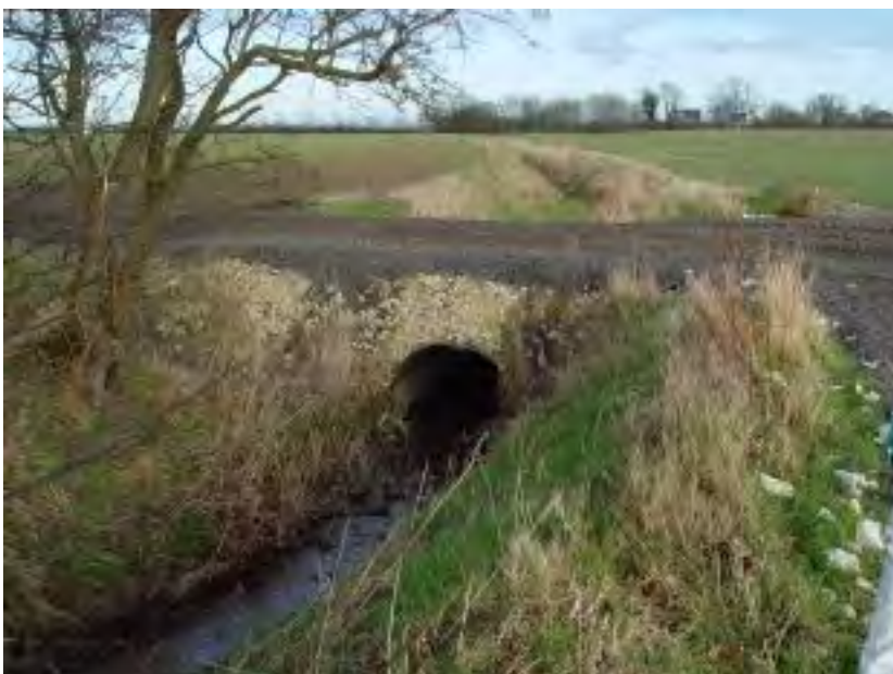
Culvert across Oldfleet Drain at the end of the wood, the track continues to the left along end of the wood towards the propose site.
