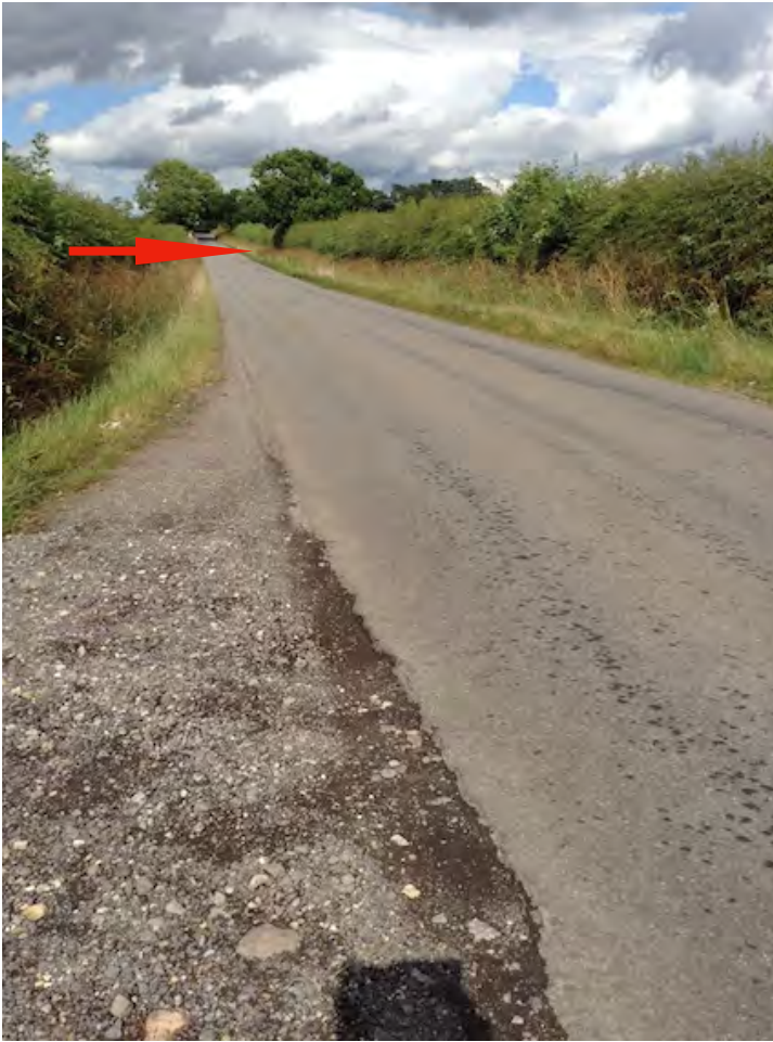
Looking toward Healing from site access. The red arrow above indicates the position of the photograph on the right.
