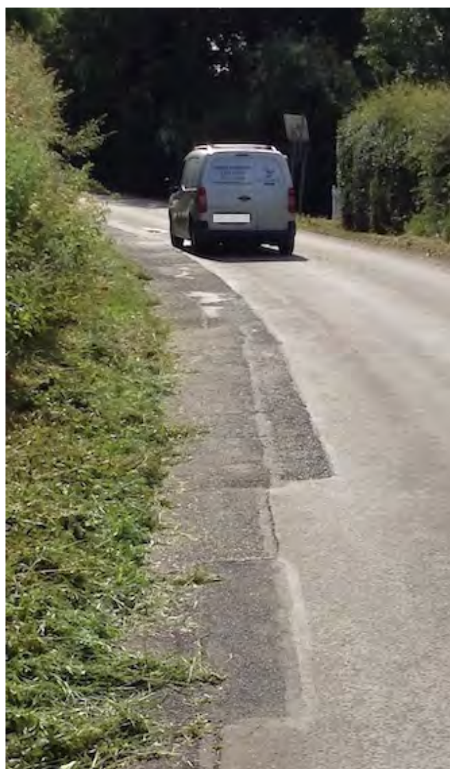
Van on blind bend, with little space with potholes on both sides of the road.
